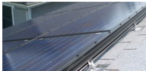
Detail of roof top solar panel installation showing mounting rails and electrical cabling
